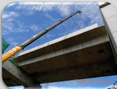
Barrier & Cable Trough
